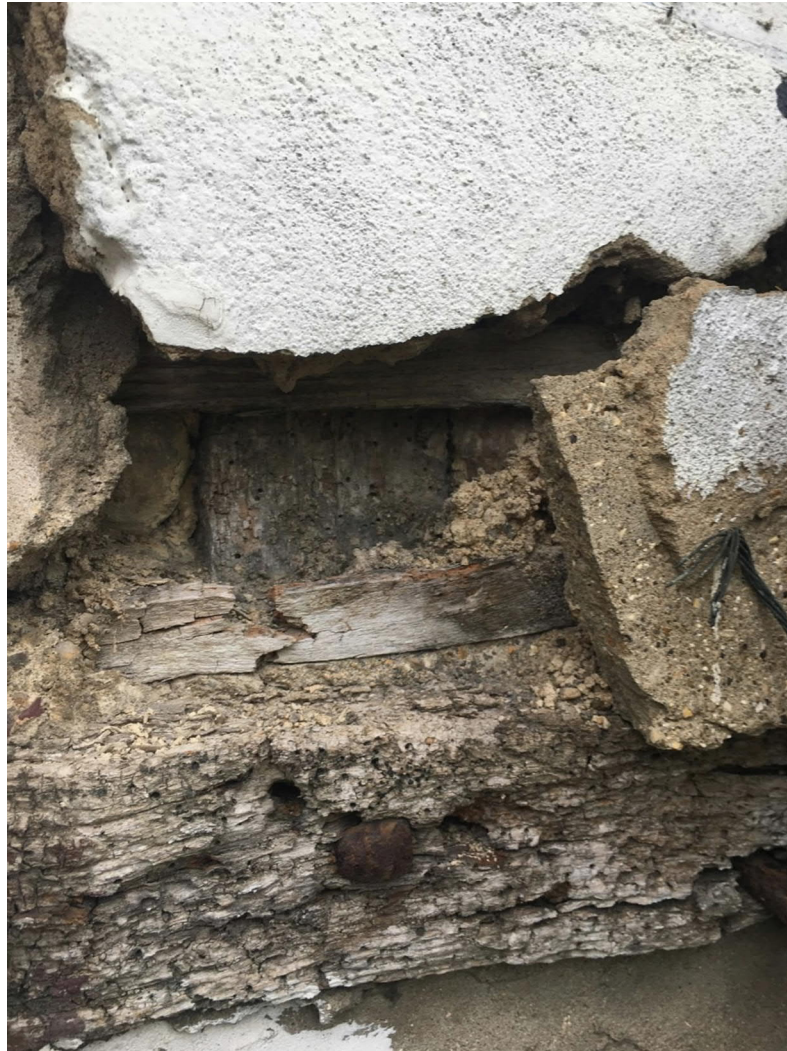
4 Damage caused by removal of pump showing remains of horizontal beam and lath and daub infill.
