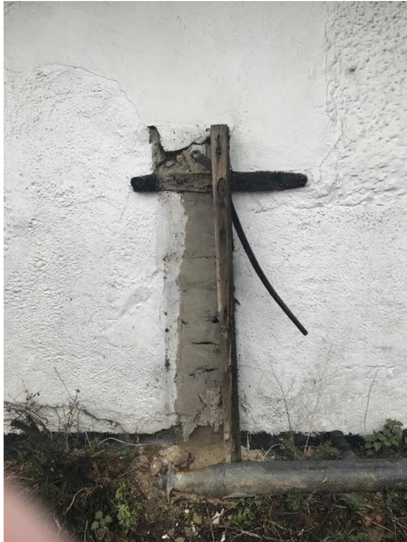
3 Remains of water pump attached to south façade. Area of cement repair below.
