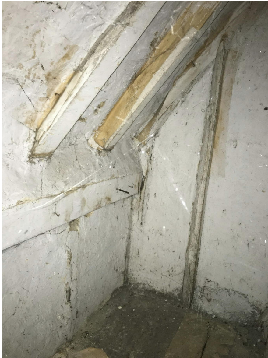
24 Framing detail visible in cupboard to north of chimney breast in no.2. Shows purlins and wall plate.
